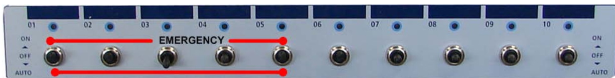
Figure 3: Emergency Relay Switches
